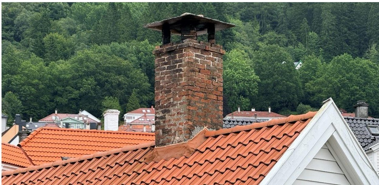
Figur 3-8 Pipe i murt tegl.
